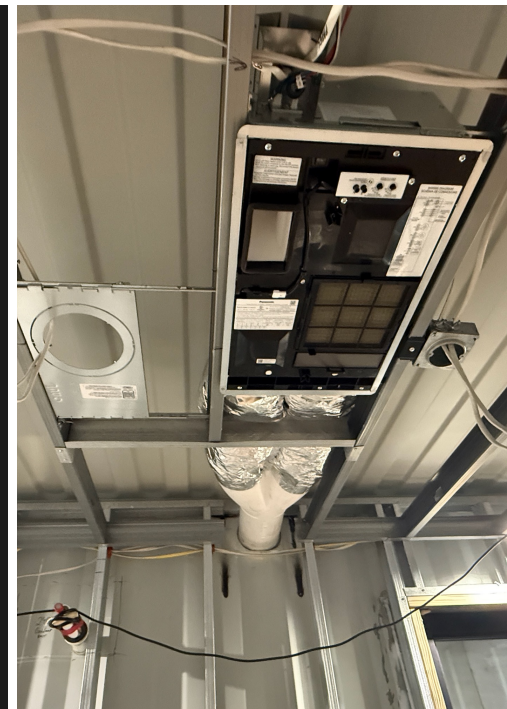
Energy Recovery Ventilation (ERV) System
